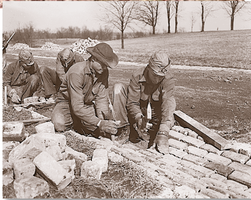
Top: This stone cabin in Chewacla State Park was built by the CCC. Above: These CCC workers are building a road.
