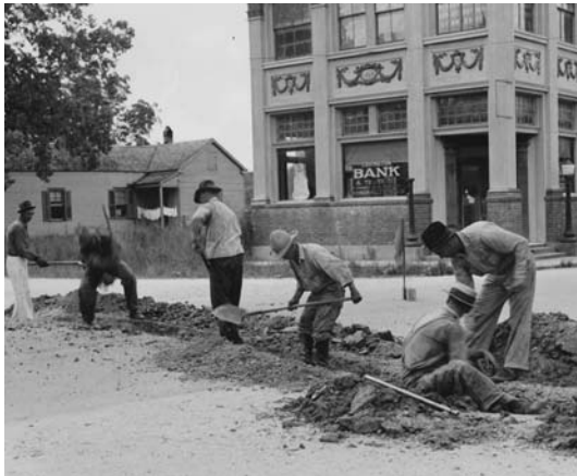
Left: WPA workers laying a water main in Madisonville in 1937. Bottom: Governor Earl Long.
